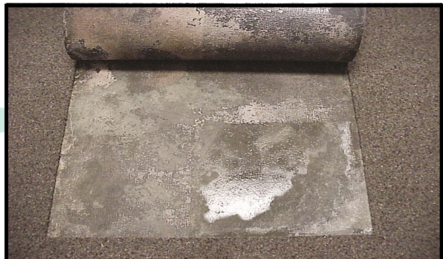
Moisture-related Floor Covering Failure (PCA image)
